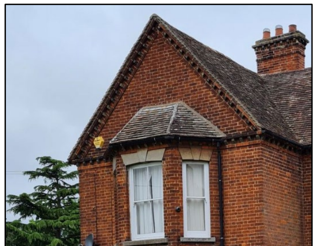
Figure 21 The 19th century addition to Lower Farmhouse, which utilises a similar dentil course within the gable end apex.
